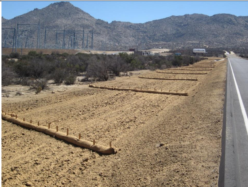
Photo 6: Erosion control measures consisting of straw wattles and hydro-mulch are being maintained along the access road to the East County Substation in accordance with the SWPPP and MM-HYD-1.
