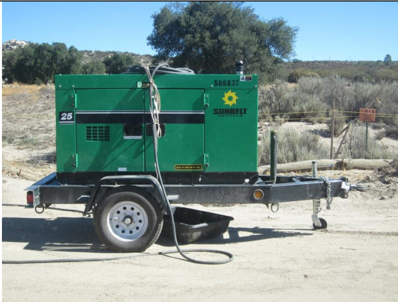
Photo 2: Drip pans were observed beneath equipment staged along the ROW in accordance with MM-HAZ-1a.
