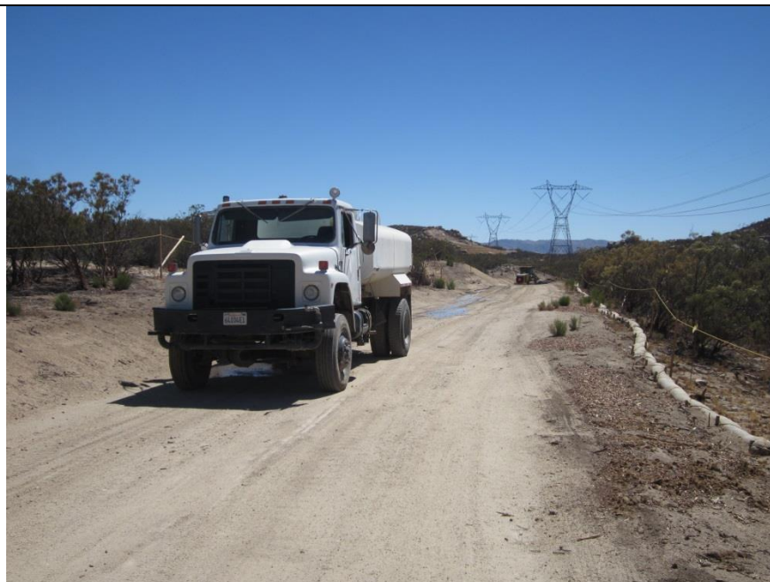
Photo 4: Water trucks were observed being utilized to minimize fugitive dust emissions in accordance with MM-AQ-1 and MM-BIO-4a.
